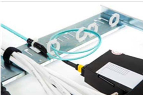
First clean MPO connector end face in the rear of the cassette, then insert the Quick-Fit MPO cassette into the UCP panel. Next clean the MPO connector end face from the incoming cable, dressing it into the cable clips at the rear of the panel (maintaining a minimum bend radius of 50mm at all times). Finally, connect the incoming MPO cable to the MPO cassette.
