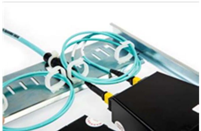
First clean MPO connector end face in the rear of the cassette, then insert the Quick-Fit MPO cassette into the UCP panel. Next clean the MPO connector end face from the incoming cable, dressing it into the cable clips at the rear of the panel (maintaining a minimum bend radius of 50mm at all times). Finally, connect the incoming MPO cable to the MPO cassette.
