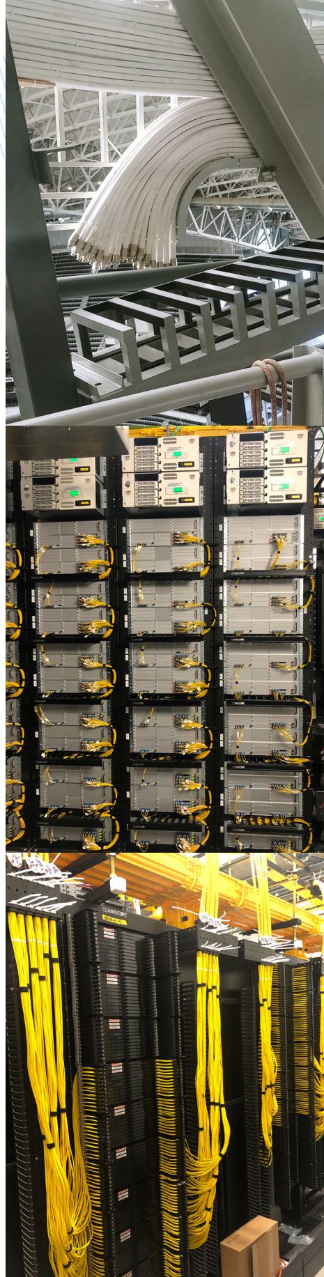
It takes a lot of wires to make a wireless network happen. Credit, top photo: ExteNet Systems; bottom photos: CommScope
