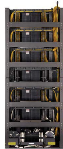
Splice chassis installed at bottom of frame (rear cover removed)
