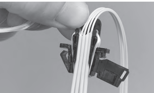
5.12 Installation of third and fourth pigtail at the opposite side of the KTU.
