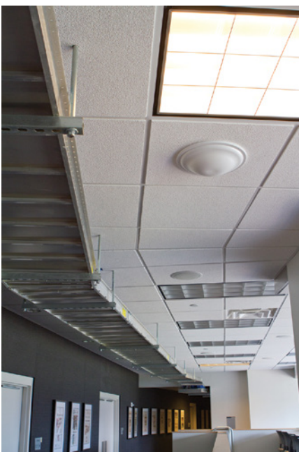
DAS Antennas at Target Field
