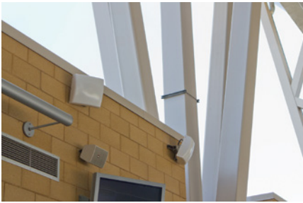
DAS Antennas at Target Field
