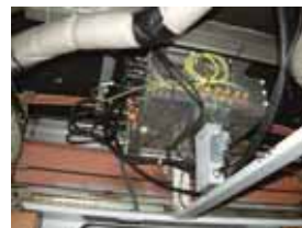
An installed in-train repeater
