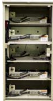
Andrew's 60ECV2 Battery Cabinet
