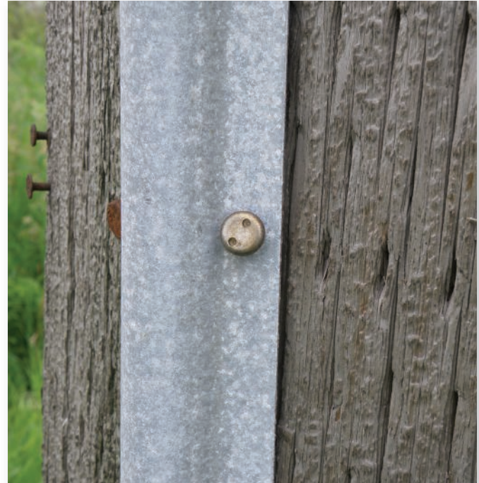
Here tamper-proof screws are used on ground wire guards.
