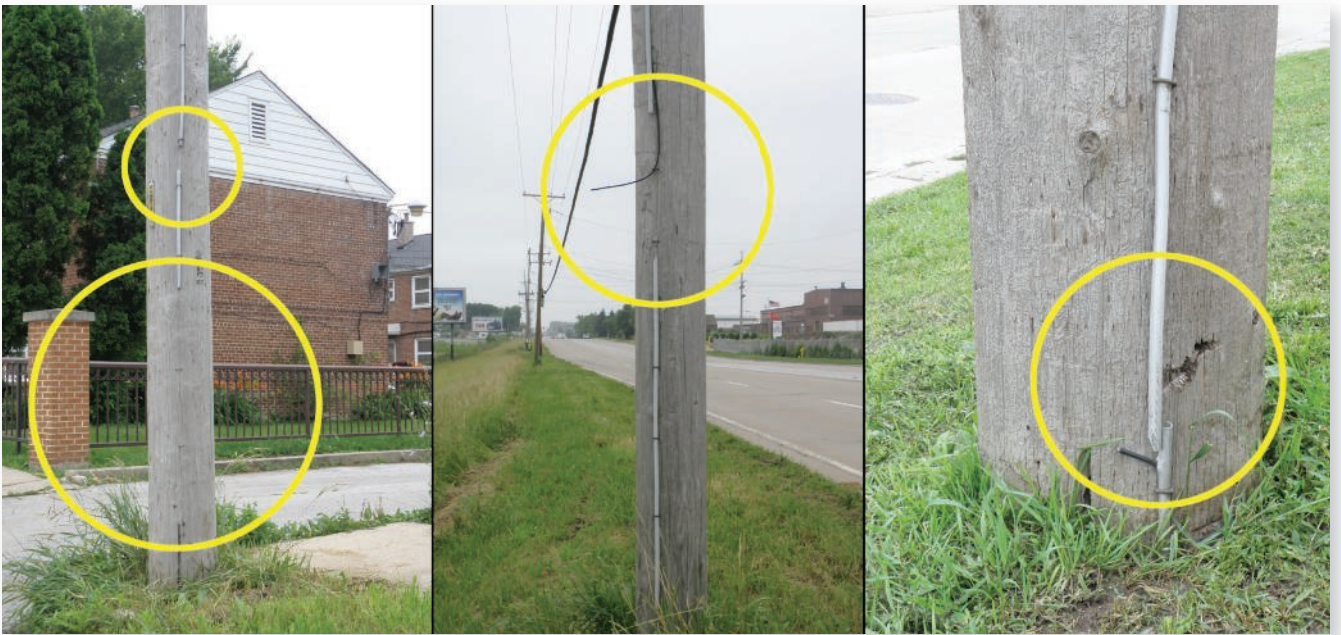
Distribution pole ground wires have long been a target of copper thieves who steal copper ground wire where it is most accessible. From left to right, ground rod cut from about 6 ft above the ground, distribution pole ground wire cut about 6 ft above the ground, and distribution pole ground wire cut at the ground line just above the ground rod.
