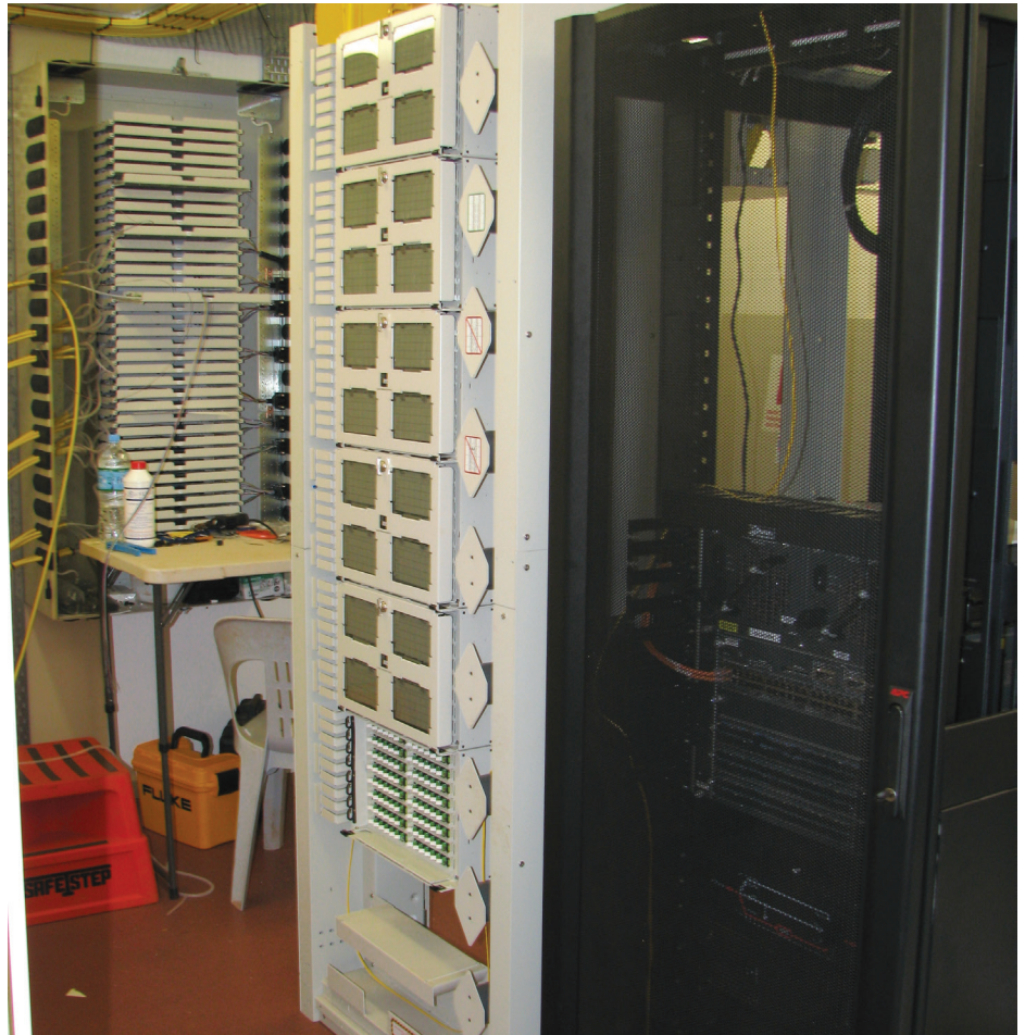
Pre-terminated fiber cables from the FL2000 Distribution Rack connect to the Fibre Entrance Cabinet for splicing to outside plant cables
