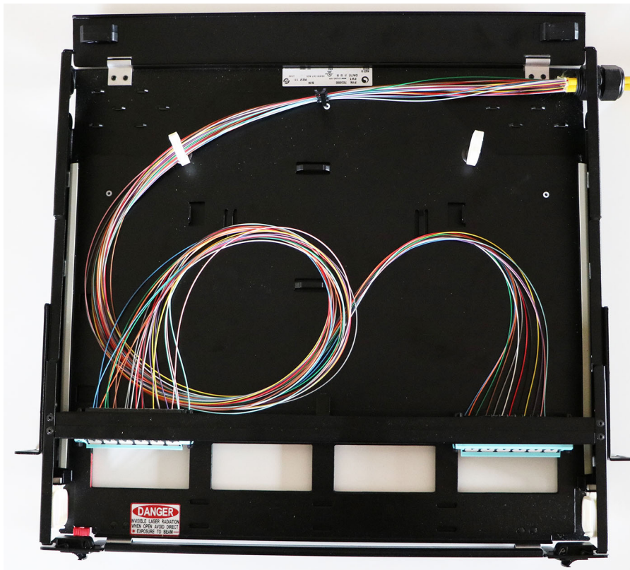
Figure 21. Cable Routing in EPX Panel
