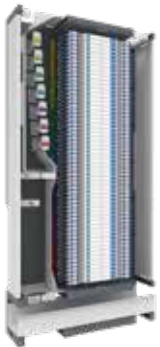
Figure 4: Single Cross Connect frame, recommended patch cord length for all cross-connects is 5 meters (17 ft).
