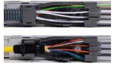
Figure 18: Installed cable termination units (CTUs) on FACT chassis
