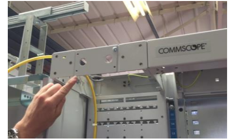
4.1.9 Fix the panel back in place and route the cable into the overhead strut
