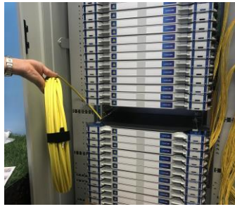
4.1.5 Unspool the cable, handle with care to avoid cable kinking
