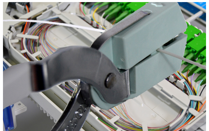
7.9. Carefully take the fibers out of the splice island. Splice the fibers to fibers that you just stripped.
