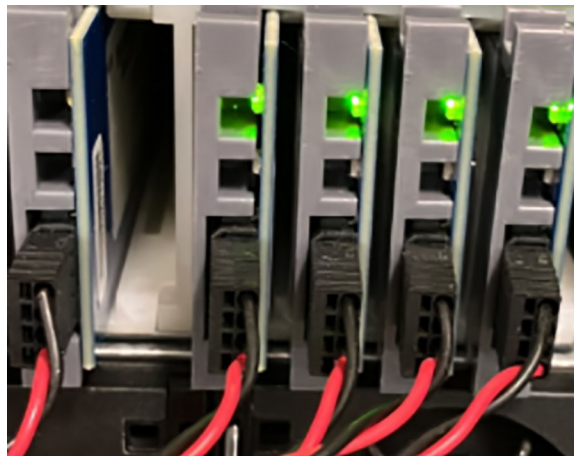
Figure 7. Transmitter End of Cable Plugged in
