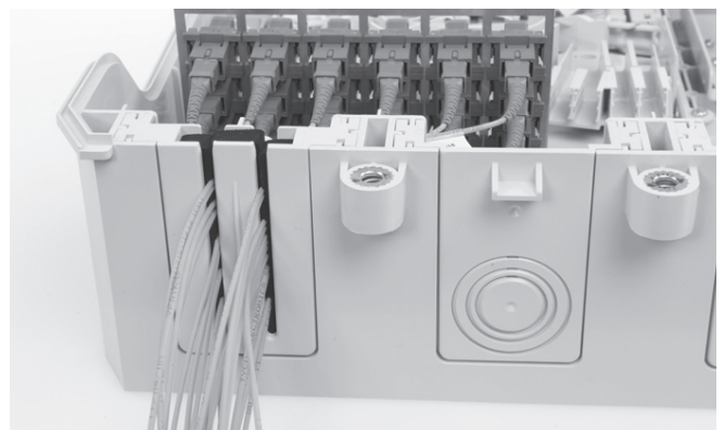
6.2 Install the next 12 patchcords and route these into the second groove of the seal.
