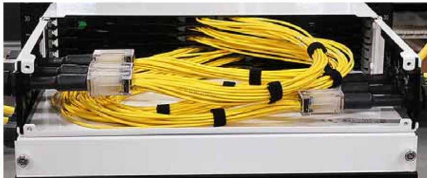
Figure 15. Cable Bundles With Hook-and-Loop Straps
