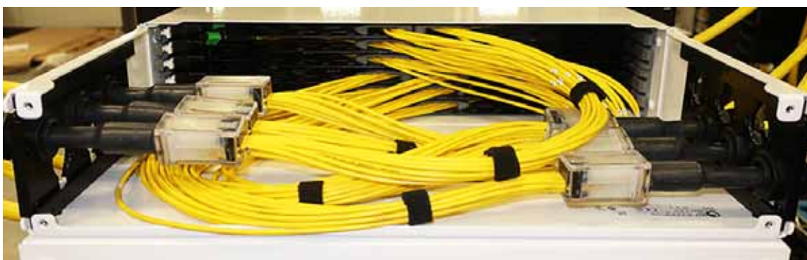
Figure 22. Cable Routing From Both Sides
