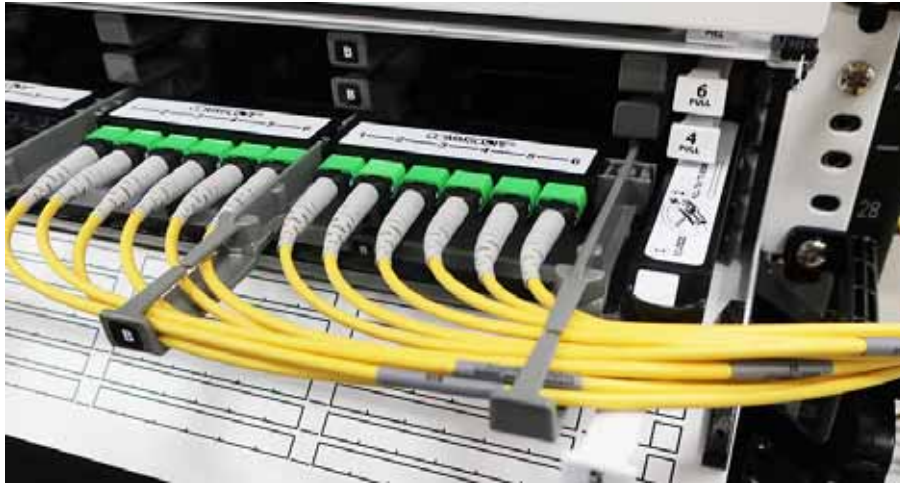
Figure 29. Patch Cord Routing on Front of Panel
